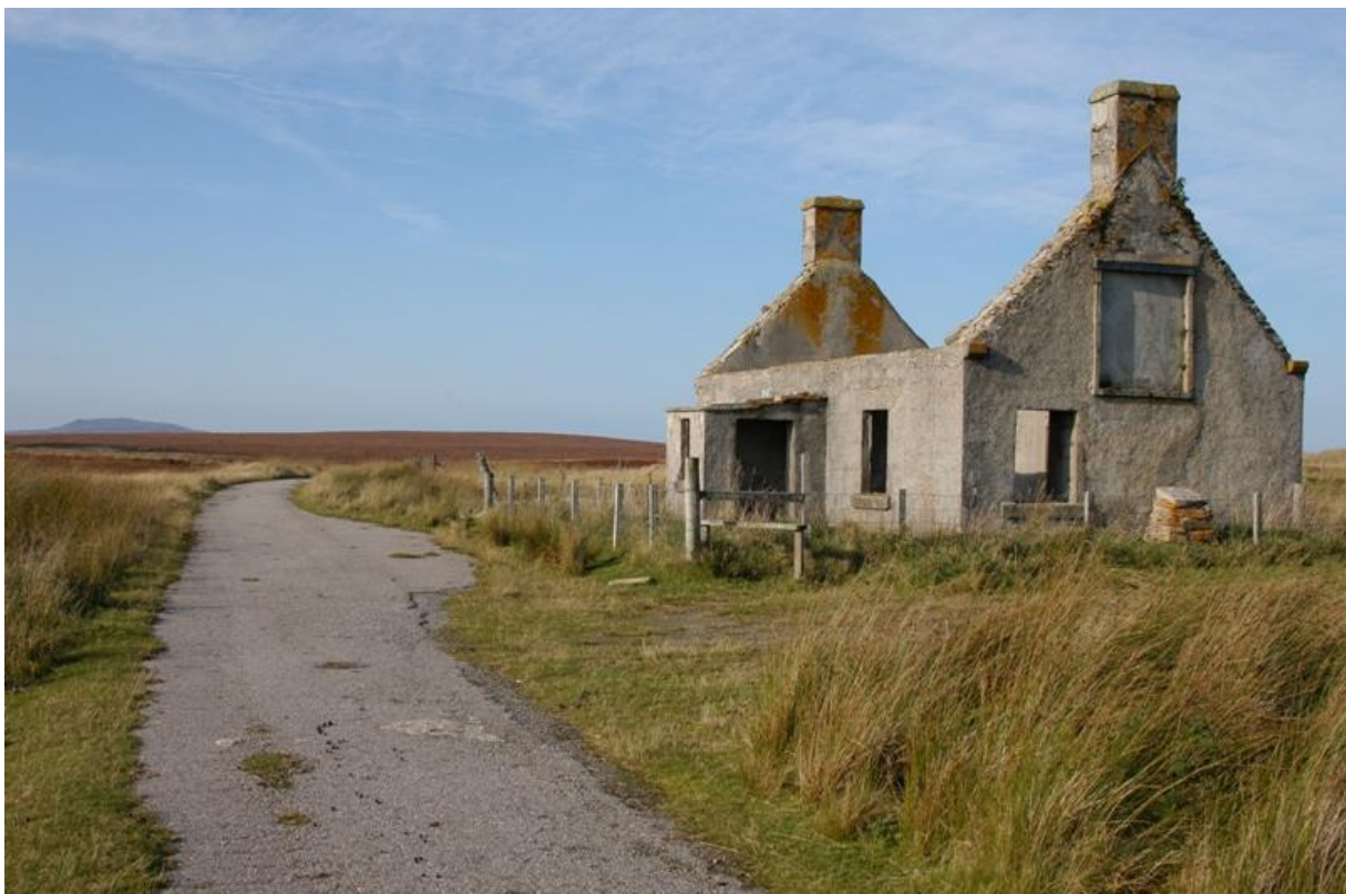
IMAGE 172 ABANDONED AND DERELICT MOINE HOUSE
